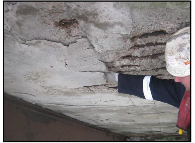
Spalling Soffit Concrete
